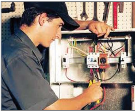
Electrician checking power board.
