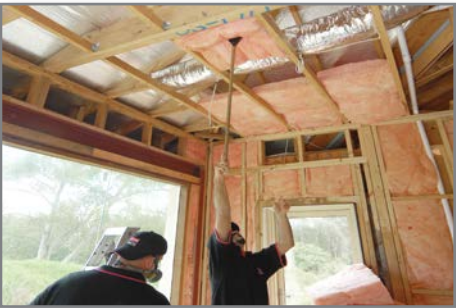
New build - Installing ceiling insulation with limited access due to ducting.
