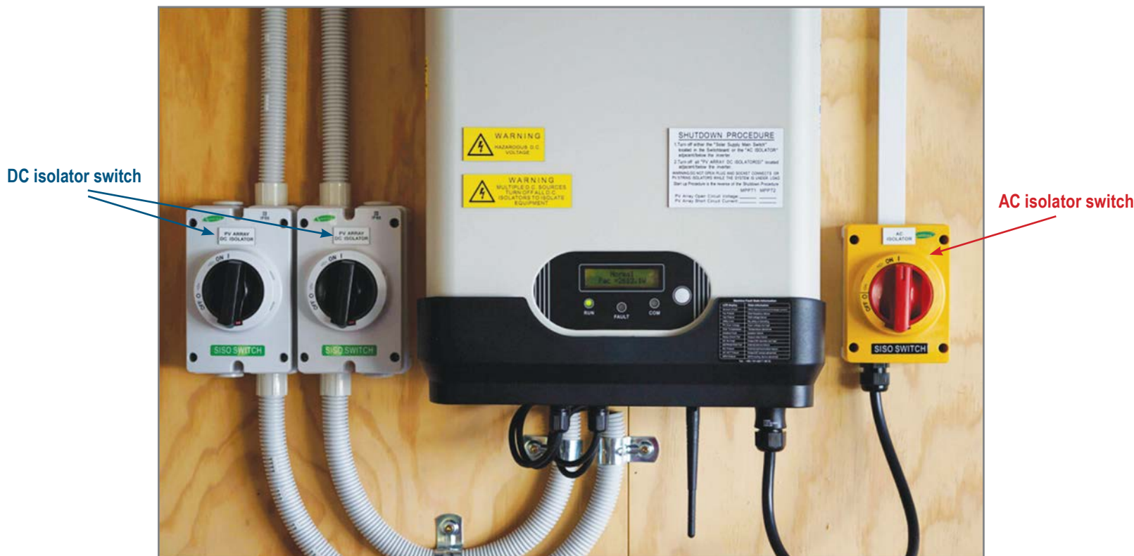
Solar Power Board
