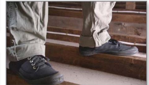
Safety: use joists for footing support
