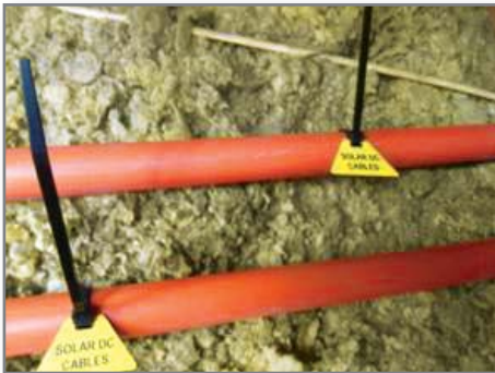
Solar Installations after 16th October 2012 using conduit to enclose wires.
