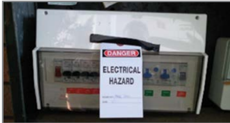
Tagged circuit board
